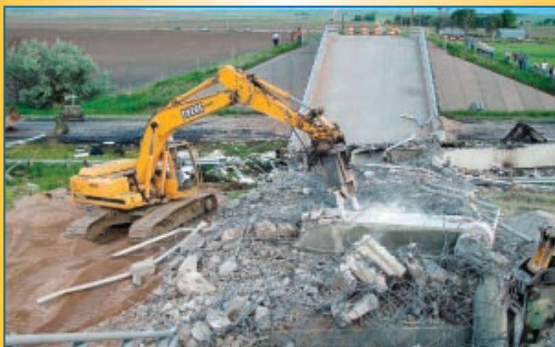
Massive cleanup begins, as crews hurry to clear I-80 of debris, and restore traffic during the busy Memorial Day weekend.
